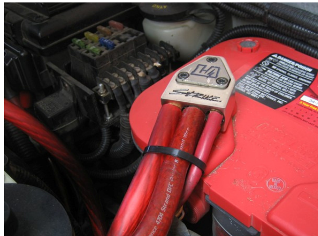
Shown are the completed connections. Note that the OEM battery clamps have been removed in favor of aftermarket battery clamps, making the connection of these VERY LARGE cables a snap.
