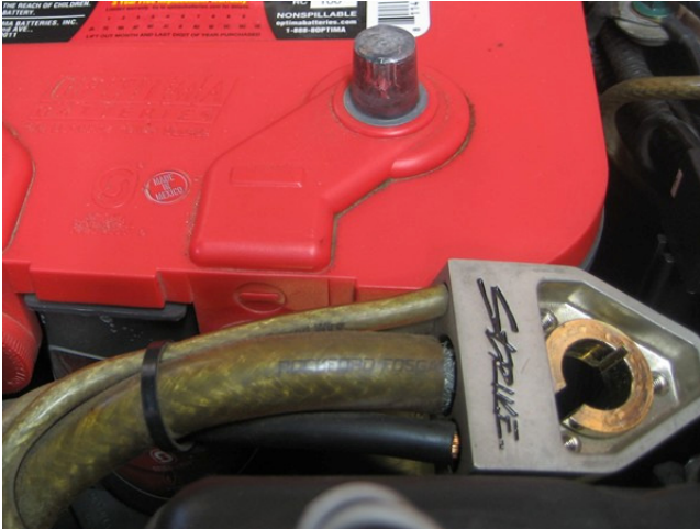
Connect the return path cable to the battery negative ( - ) terminal. Note the use of an aftermarket battery clamp to facilitate this.
